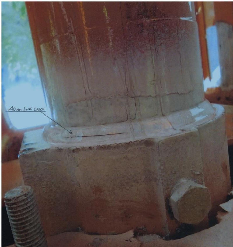
40mm long crack
