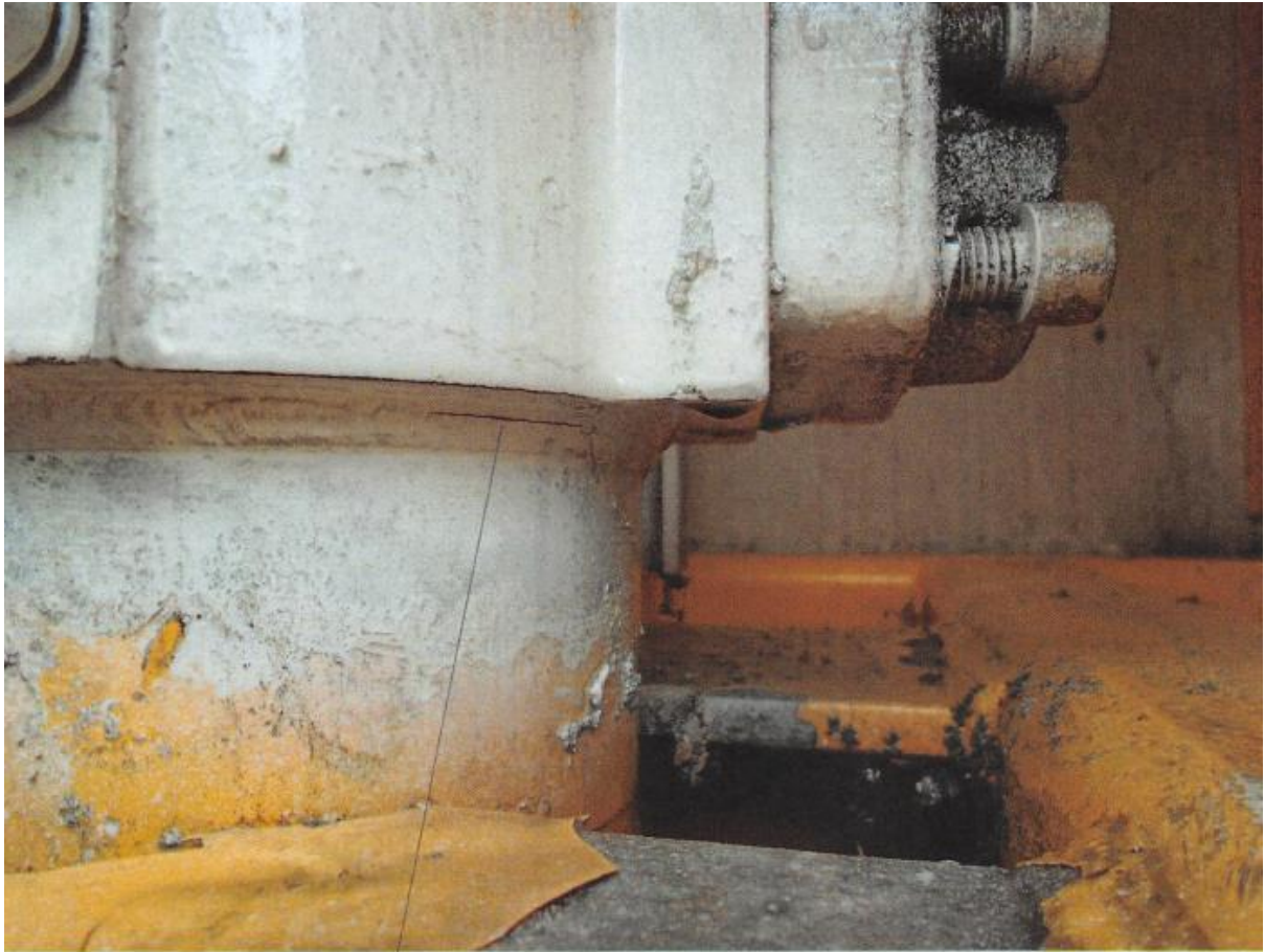
25mm long crack revealed by MPI
